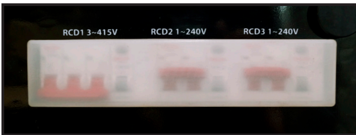
RCD protection for all high voltage circuits
